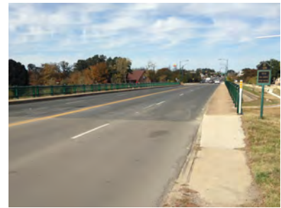
Pedestrian safety along the bridges are a major concern.
