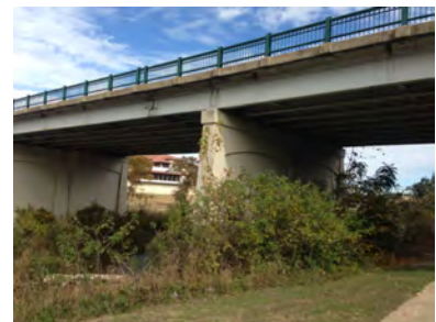
Repairing the bridge superstructure is needed.
