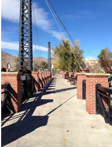
The sidewalk passes under the cables and the towers present playful shadows on the concrete deck.
