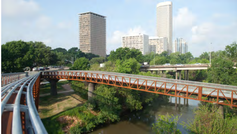
The bridge railings are made of galvanized steel which contrasts with the corten steel truss structures.
